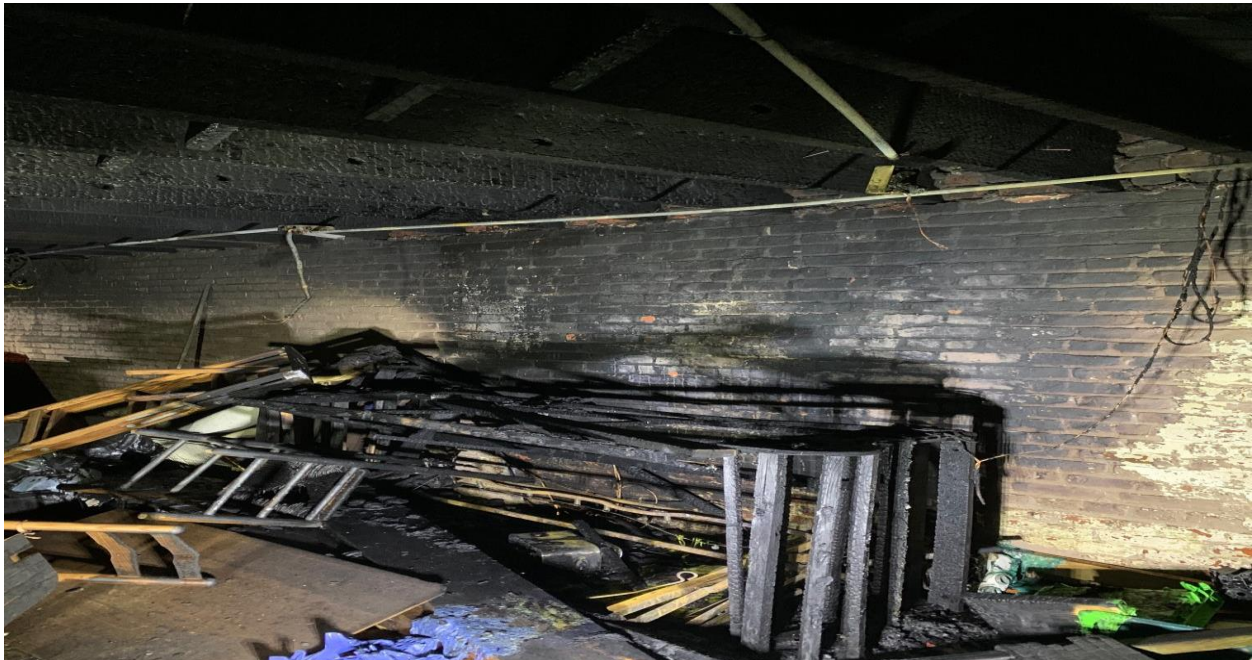
Origin & Cause Investigation (Overloaded Extension Cord with V-Pattern)
