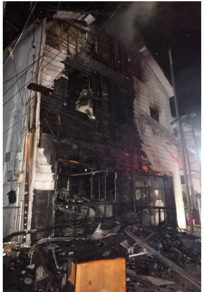
Vacant structure fire at 669 Charles Street on the Night of October 10, 2016
